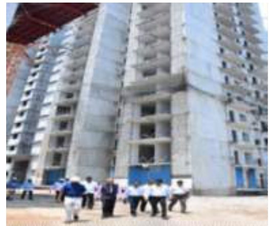
Residential Flats by using Monolithic construction technology with tunnel form shuttering at Chennai
