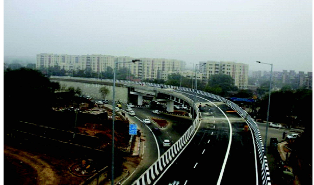
Newly constructed Flyover and Underpass completed just in 13 months against stipulated completion of 24 months with saving of Rs. 26 Crore
